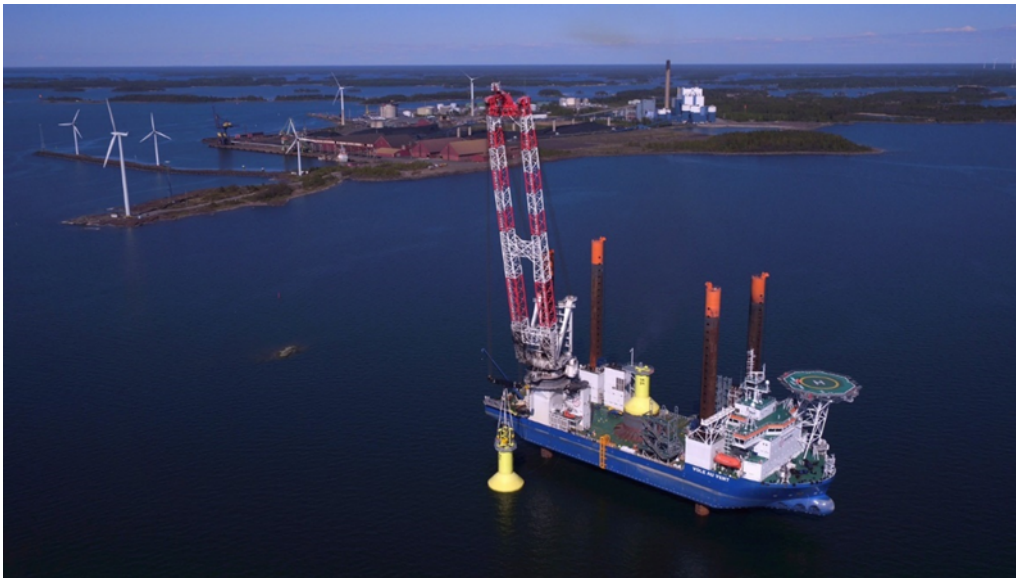
Figure 6-4: Gravity-based Foundations Transported on Vole au vent Offshore Jack-up Installation Vessel (Credit: Jan De Nul Group)
