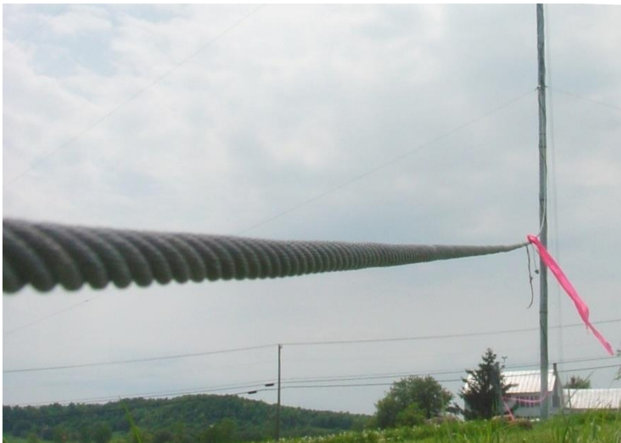
Picture 4-8: Level 1, guy sag = 2.5 tubes - too loose
