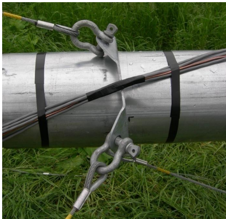
Picture 3-29: Cable protection
