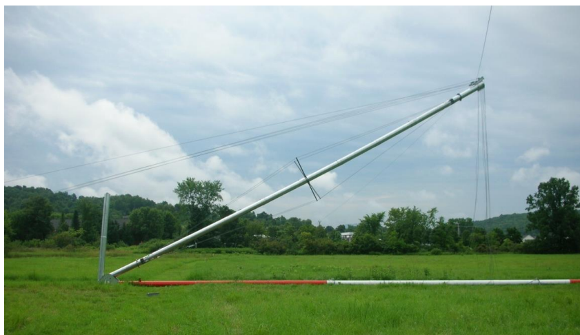
Picture 4-1: Correct time to check for winch cable twists-if all is good, remove the helper ginpole
