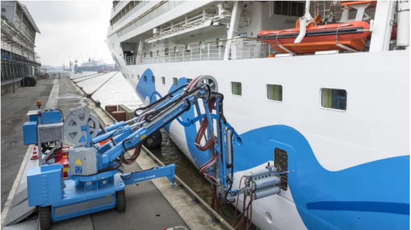
Shore power at the Port of Hamburg (BBC 12 )
